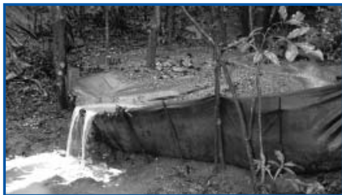
Silt fence during rain, demonstrating the large amounts of sediment washing into the Francis Bay wetland.
